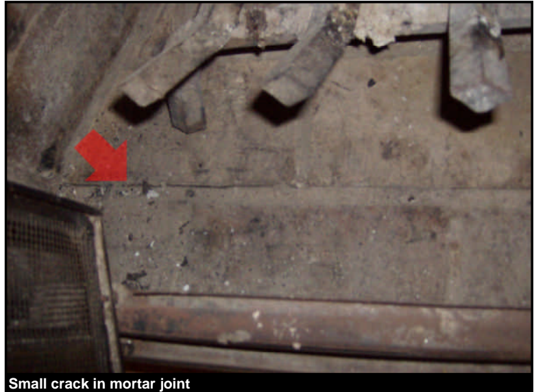
Small crack in mortar joint
